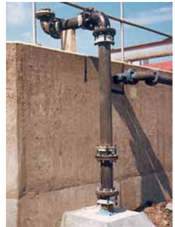
118mm FlexLock flange adaptors installed on Ductile Iron pipework.
